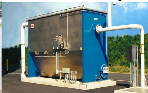
Above ground oil separator
